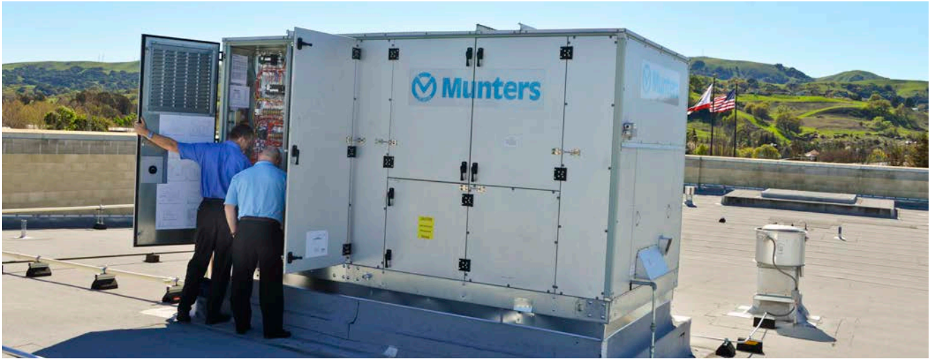
Indirect Evaporative Dedicated Outdoor Air Unit field testing at Whole Foods in San Ramon, CA.
