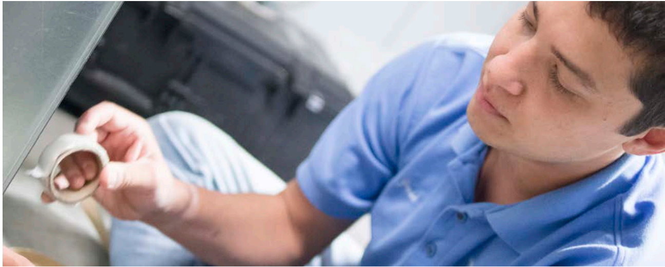
Jose Garcia, WCEC Assistant Engineer, sealing ductwork for WCEC's laboratory environment chamber.
